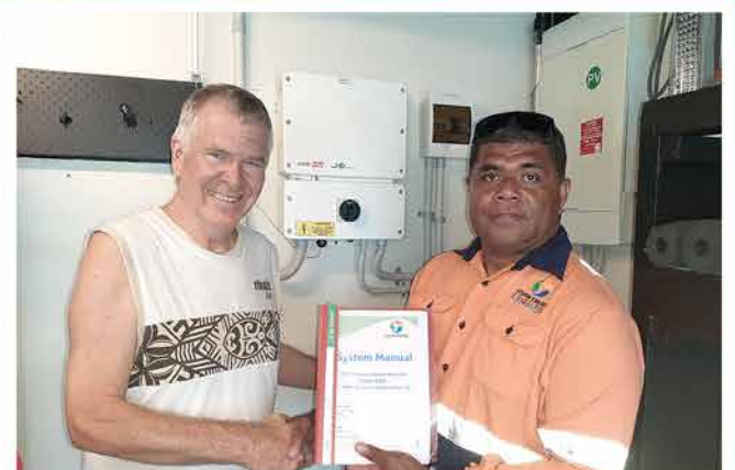
Residential Solar System at Pacific Harbour
